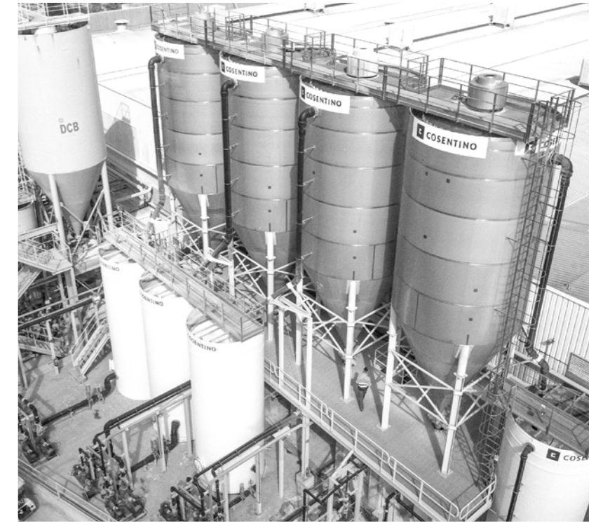
→ Water Recovery Plant
